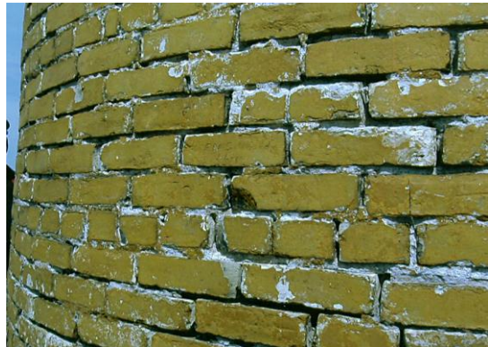
Rear Range Light outside brick damage
